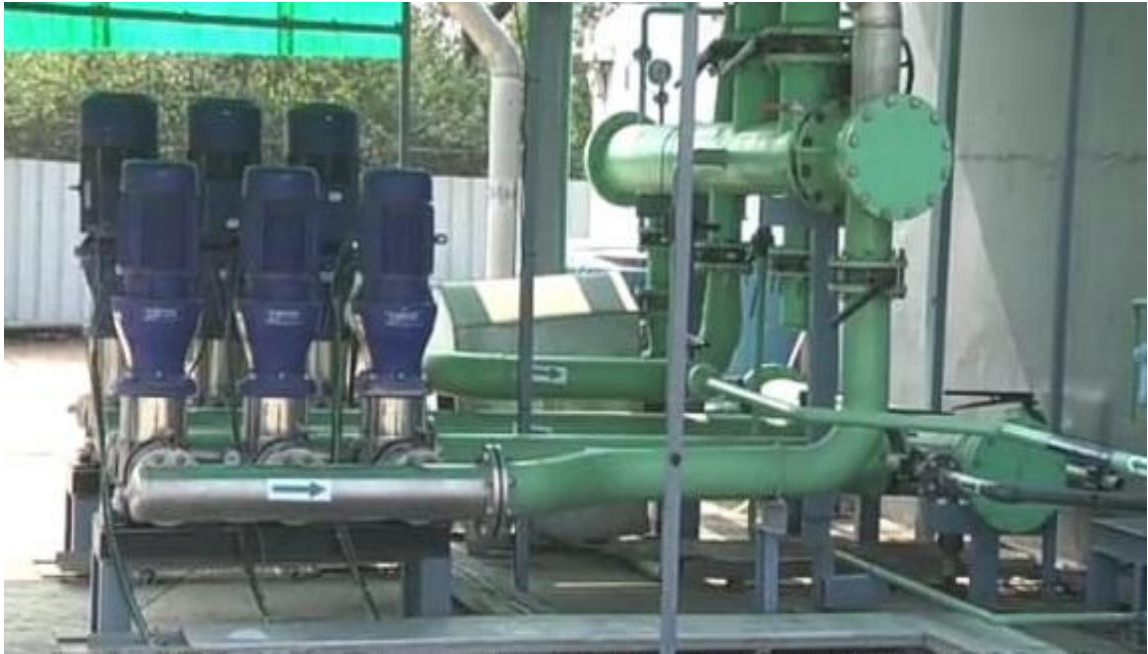
Treatment and Distribution
